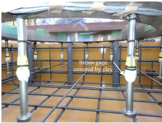
Fig. 5 – Strain gages on anchors
