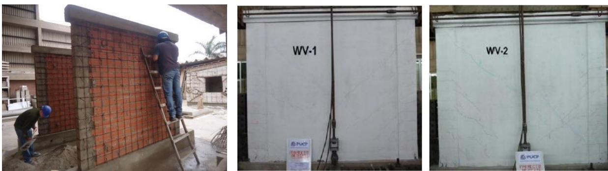
Fig. 6 – Confined masonry walls retrofitted with wire meshes, subjected to vertical load and cyclic lateral load [13].
