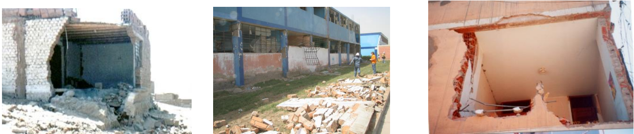
Fig. 8 – Collapse of masonry walls due to poor construction and deficient design.
