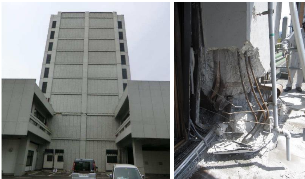
Fig. 1 – (Left) Overview of Building of Faculty of Architecture and Engineering at Tohoku University (from Wang, 2014), and (right) damage observed to a boundary column after the 2011 Tohoku Earthquake.
