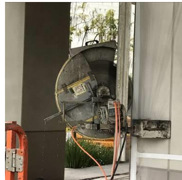
Fig. 13 corner joint widened by sawcut
