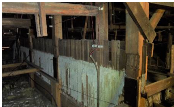
Fig.10-Lath wall that is not reached to the beam
