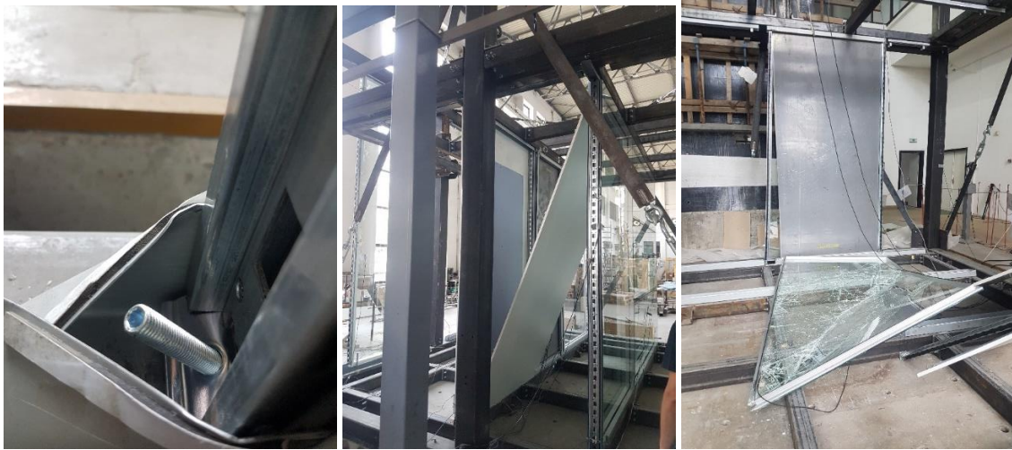
Fig.10: Photos showing damages of partition walls
