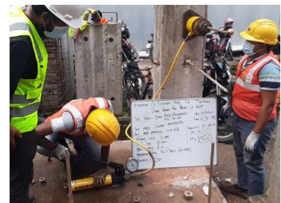
c) Pullout on column
