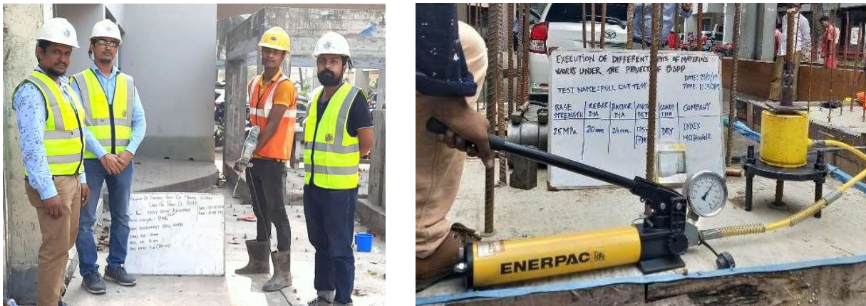
Fig. 1 – Pullout test set up at site. a) Work group, b) Pullout test machine
