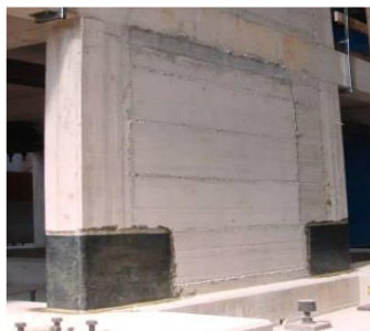
Fig. 2 – Three-sided CFRP jackets to reinforce the edges of the wall on the ground floor. [8]
