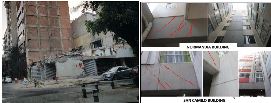
Fig 1 - (a) Collapse of a building with discontinuities; (b) Diagonal Cracks in the beams of the transfer floors in two buildings supporting six and seven levels respectively.
