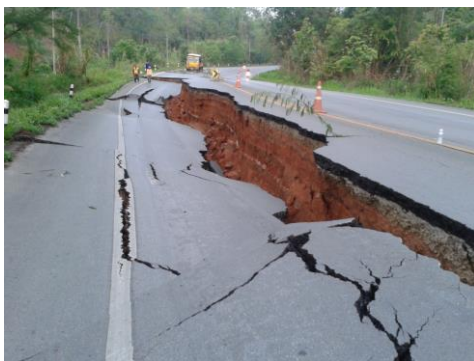
Fig.1- Failure of a highway embankment
