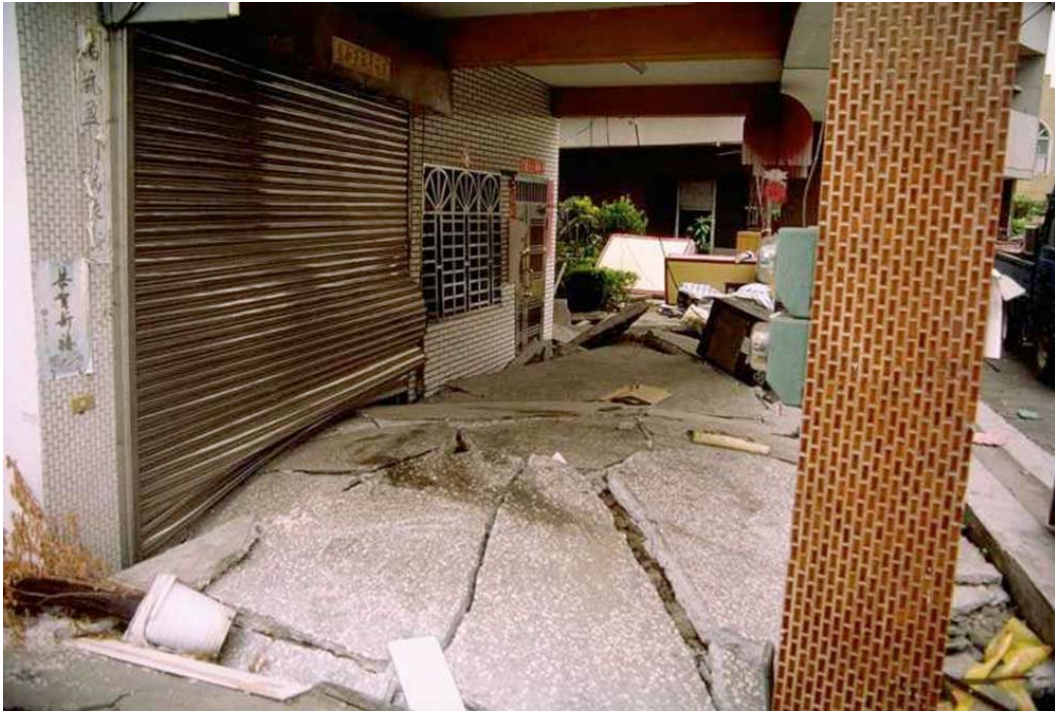
Fig. 1 – Punched footings and intermediate slab heaving due to cyclic softening of high-plasticity clay in Wufang, Taiwan. Photo by R. Seed (1999).
