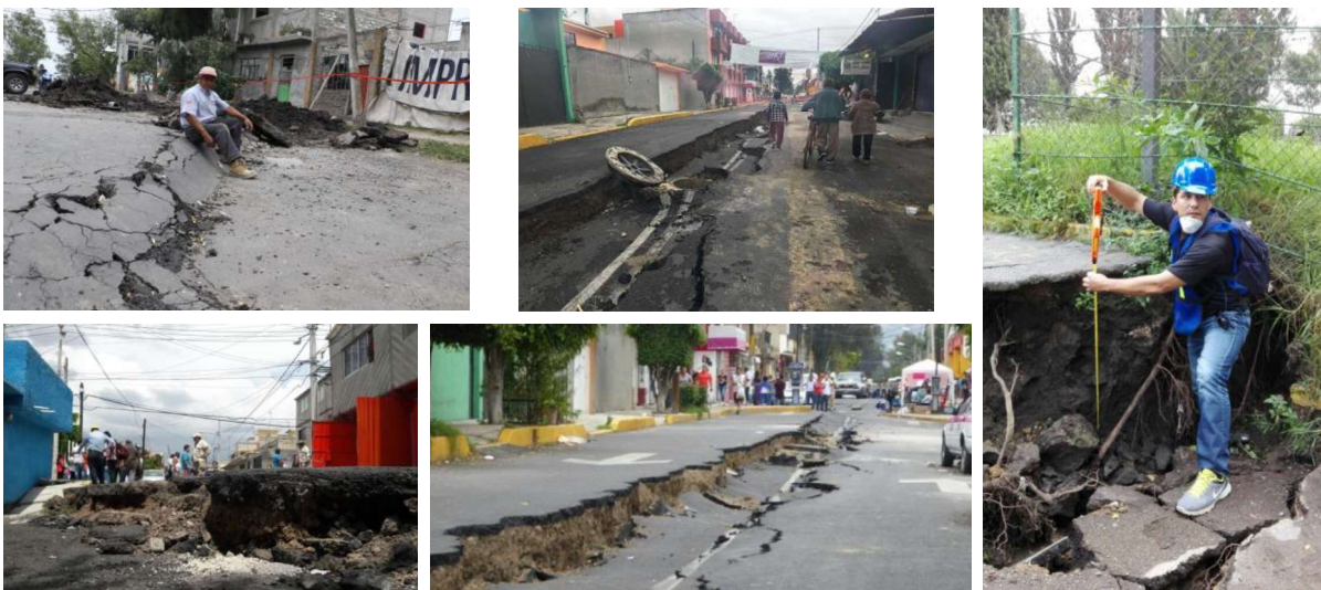
Fig. 5- The sinking phenomena and the derived effect on soils of the southern region in the City: cracking.
