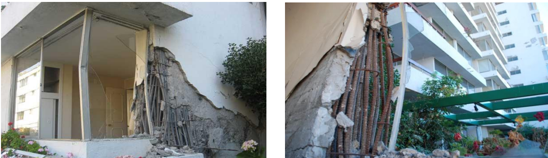
Fig. 9. Damage patterns in Viña del Mar
