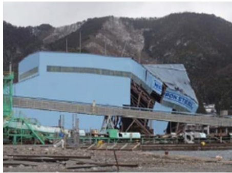
Fig. 1 An example of building collapse due to tsunami-driven ship collisions [1]
