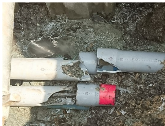
Fig. 2 An example of damage
