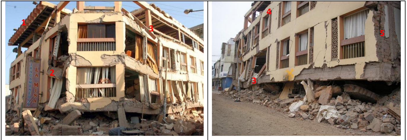
Figure 5: External Assessment . Numbers correspond to hazards shown in the images and table.
