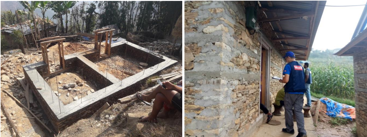
Figure 7. Construction of a house up to sill level, left; inspection of completed walls, right.
