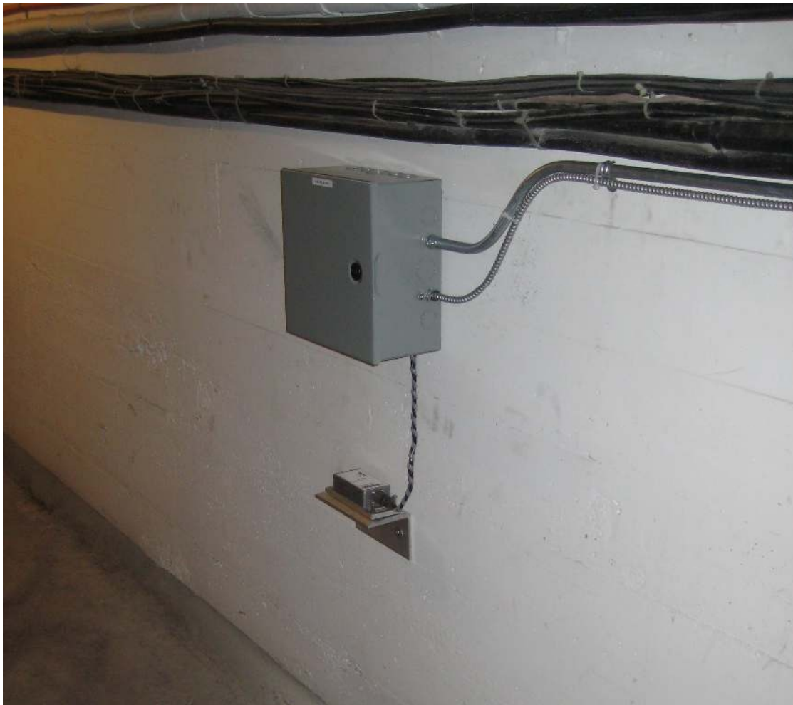
Fig. 2 - PPR Sensor mounted on a foundation wall
