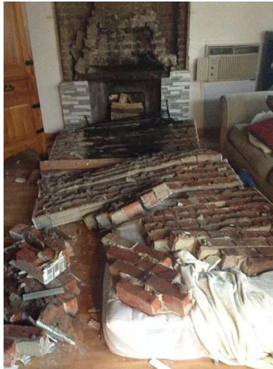
Fig. 10– Fireplace surround that peeled off the wall seriously injured a 13 year old boy in the 2014 South Napa Earthquake (California, United States). (Photo credit: ABC7 News)
