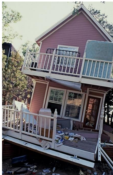
Fig. 6– Two-story wood-framed house that slid down the hill during the 1992 Big Bear earthquake (California, United States) sustaining significant damage to the superstructure. (Photo credit: California Office of Emergency Services, CalOES)
