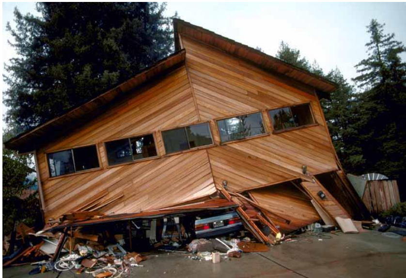
Fig. 4— Single-family wood-framed house with the living-space-over-garage vulnerability severely damaged in the 1989 Loma Prieta Earthquake (California, United States). (Photo credit: FEMA)
