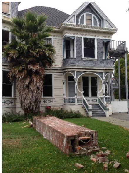
Fig. 8– Unreinforced masonry chimney pulled away from the house in the 2014 South Napa Earthquake (California, United States). (Photo credit: CEA)
