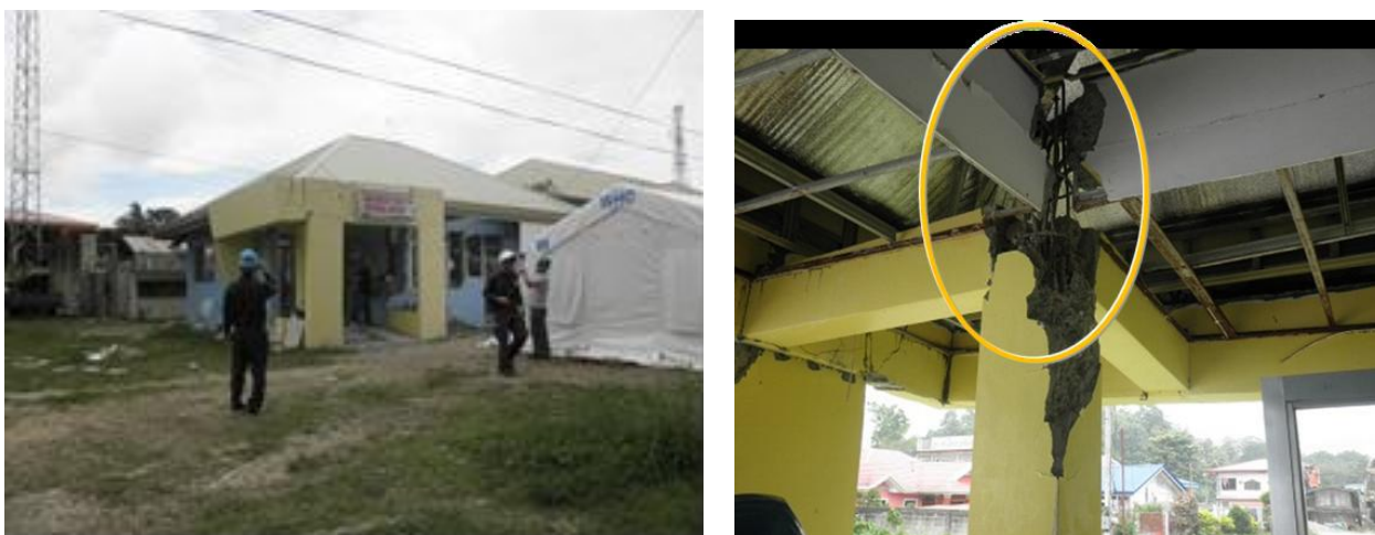
Figure 1 An example of improper structural design: (Left) Exterior view of District Health Care Center of Sagbayan, (Right) connection of a column and beams at different level, which might cause the failure because of local strong stress
