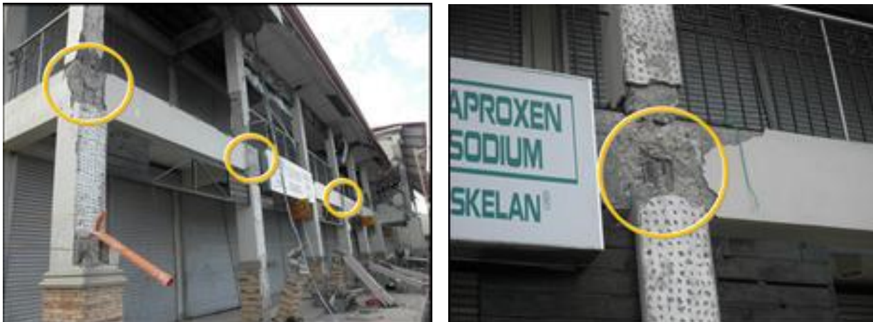
Figure 3 An example of improper rebar works in Market Building in Loon: (Left) Failures at panel zones (joints of columns and beam), (Right) Detail of damaged part. Hoops are not installed at the panel zones.
