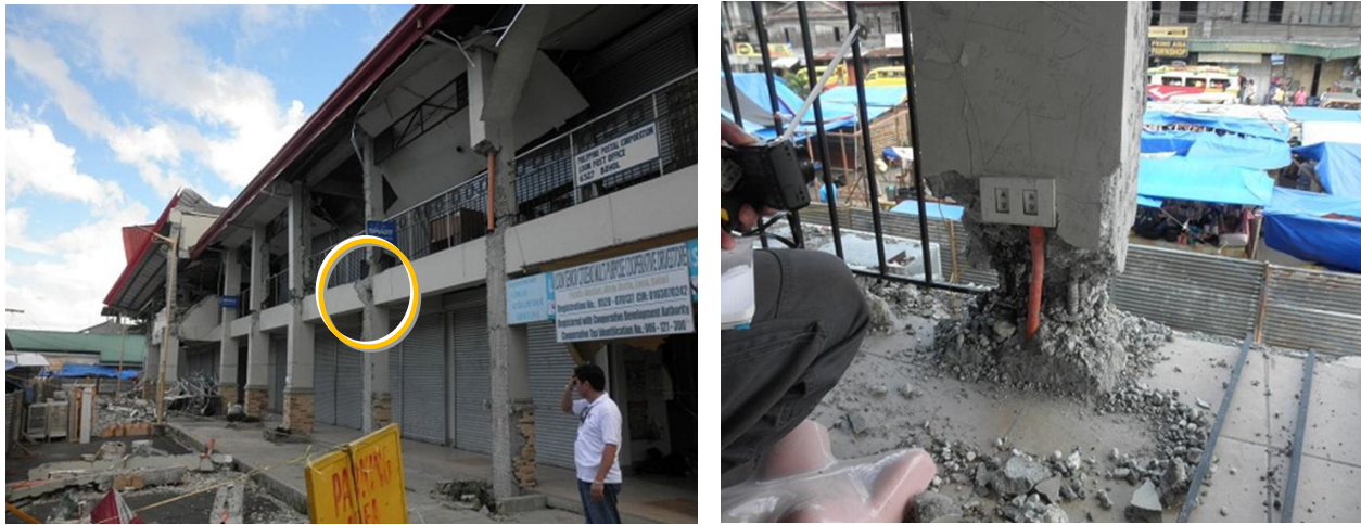
Figure 2 Examples of serious damage in columns in Market Building in Loon: (Left) Heavy damage at the bottom of most of columns, (Right) Detail of the damage. The causes may be improper casting and insufficient compaction of concrete, congestion of rebar caused by concentrate of overlapping splices, and imprecise positioning of longitudinal rebar.
