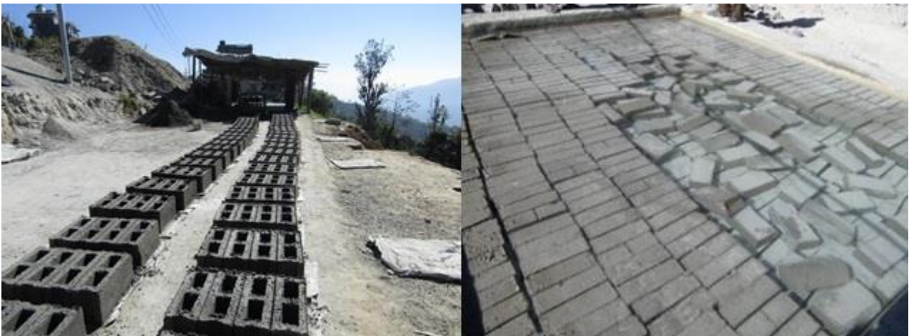
Fig. 4 – HCB laid in the sun after production in Dolakha (L) and blocks submerged in a pond in Dolakha (R).
