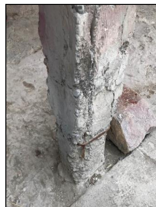
(b) Inadequate cover of a column and exposed rebar
