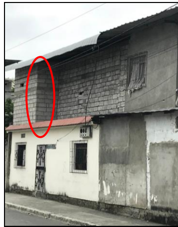
(b) Column absence
