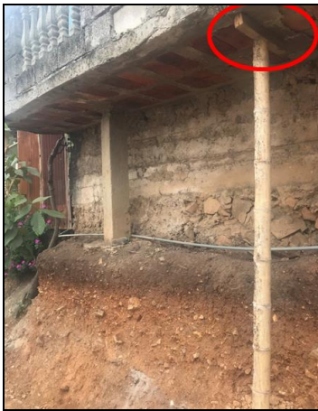
(a) Missing structural element
