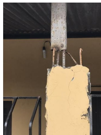
(b) Inadequate connection column - roof
