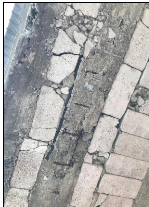
(a) Inadequate beam cover and exposed rebar
