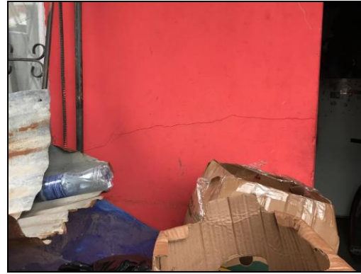
(b) Non Structural damage between openings
