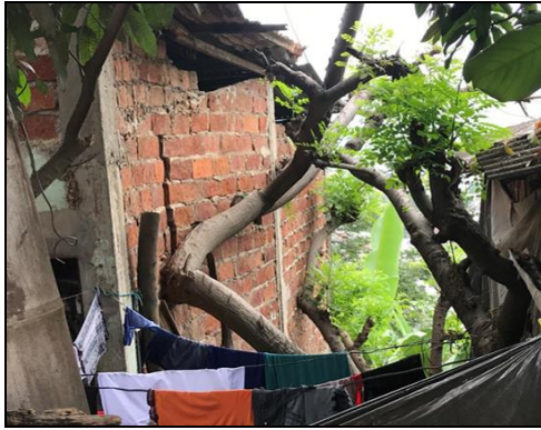
(a) Non Structural damage caused by a tree
