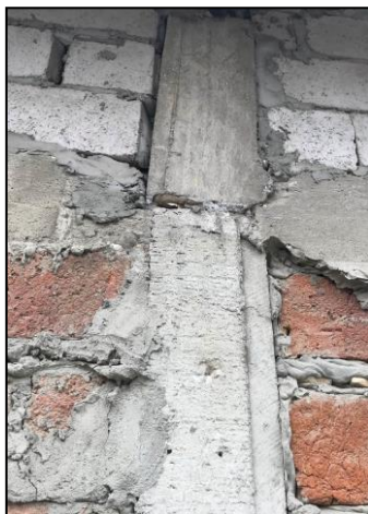
(a) Inadequate connection column - beam
