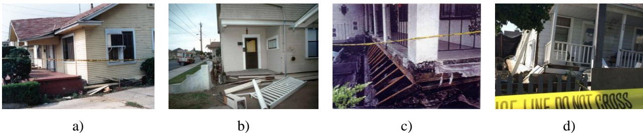
Fig. 1 – Examples of unbraced cripple wall failures following earthquakes: a) 1987 Whittier (Photo: Whittier Museum), b) 1989 Loma Prieta (Photo: USGS), c) 1994 Northridge, d) 2014 South Napa (Photo: LA Times)
