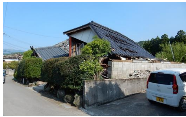
(b) Severely damaged SFD near solar farm
