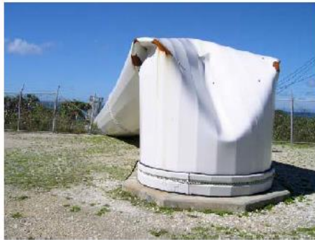
Fig. 5 – Tower failure caused by local buckling (400 kW capacity turbine, Japan, 2003) [4, 5]
