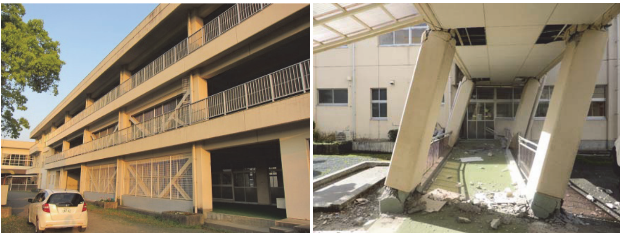
Photo 4: Survived and severely damaged school buildings (2016 Kumamoto earthquake) [7]
