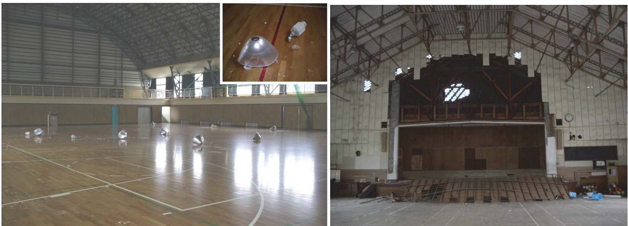
Photo 2: Structural and non-structural damage to school buildings (2004 Niigata-ken Chuetsu earthquake) [5]
