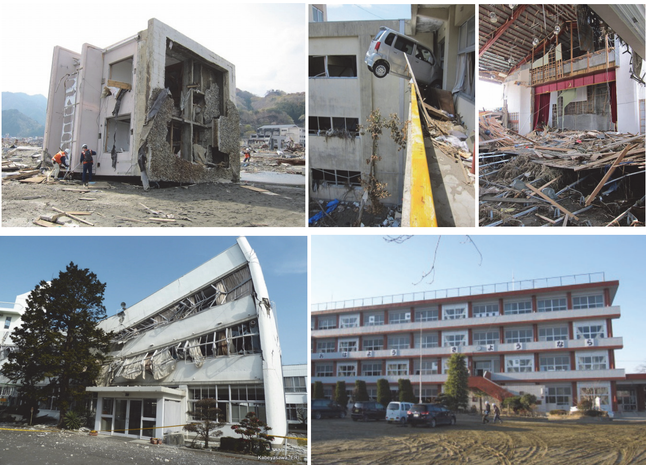
Photo 3: Ground shaking and tsunami damage to school buildings (2011 Great East Japan earthquake) [6]
