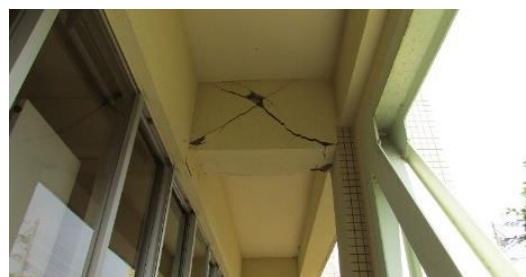
Fig. 2 – Failure situation of the beam in the short direction
