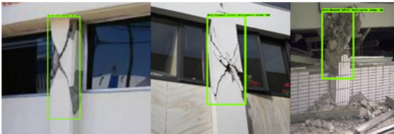
Figure 6. Bounding box classification results: shear damage to short/captive column.
