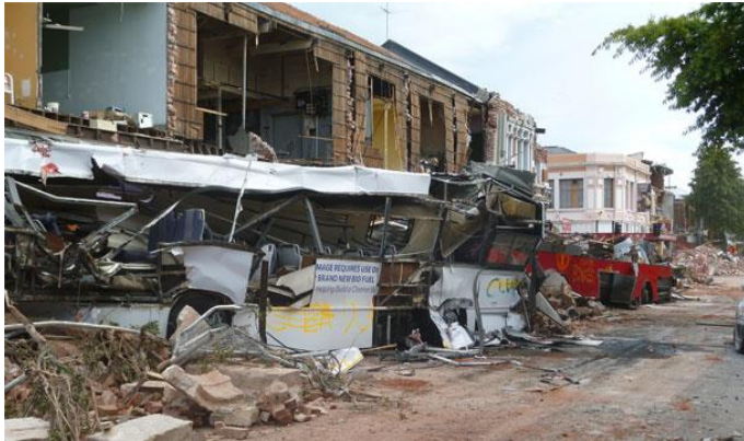
(a) Example of out-of-plane wall failure from Christchurch earthquake [5].
