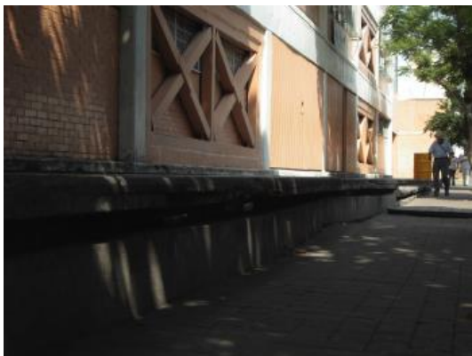
Figure 4 The separation between the foundation and the building
