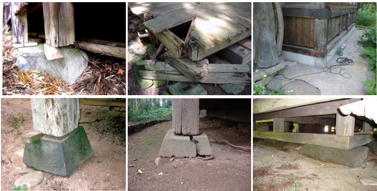
Figure 2. Details of the damages at the bottom of columns
